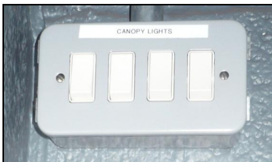
Exterior Canopy Lighting Clearly Labelled
